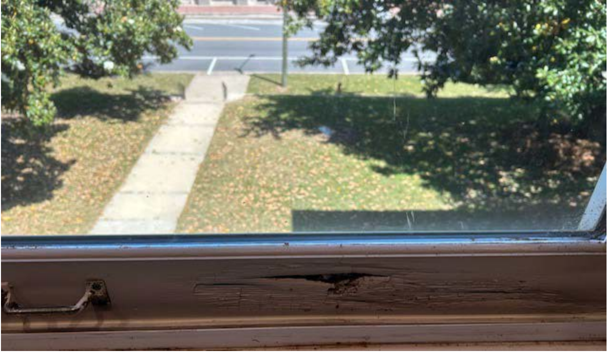
Interior wood damage due to deterioration
