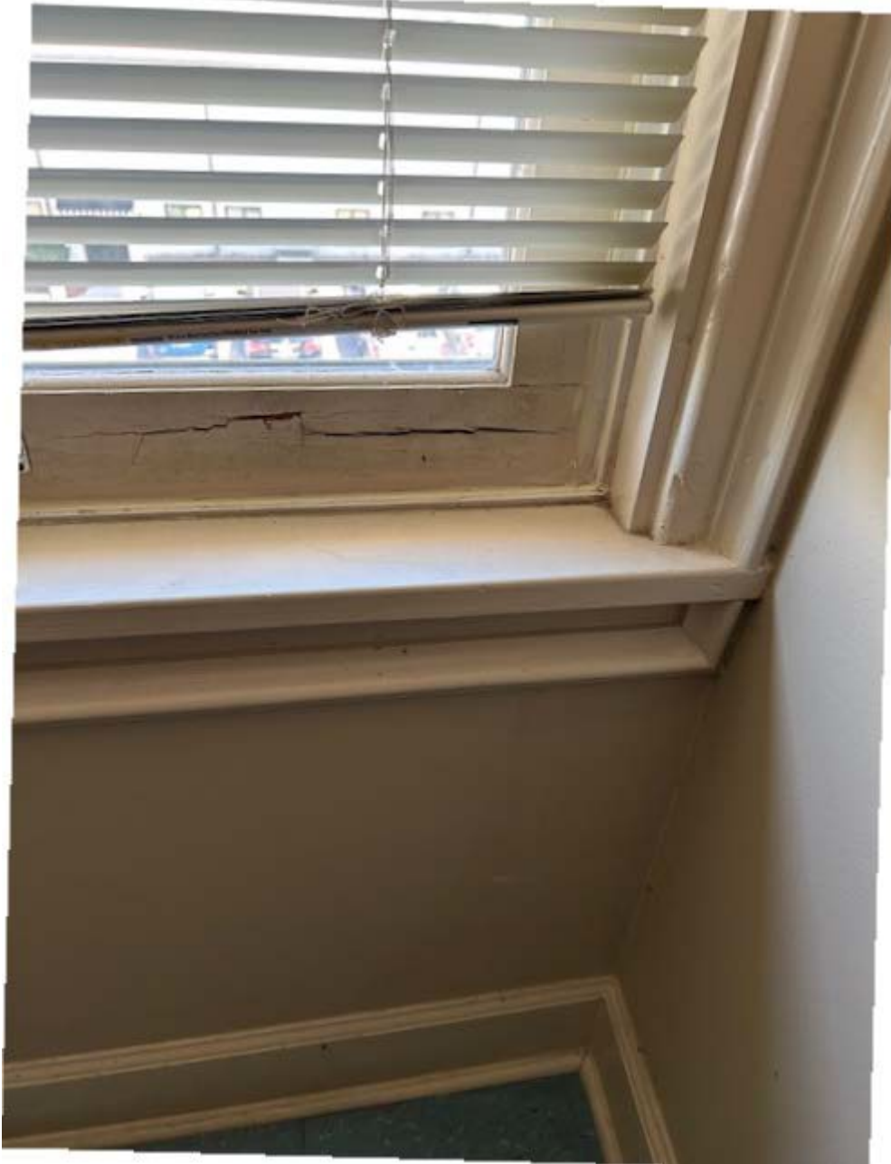
Interior wood damage due to deterioration
