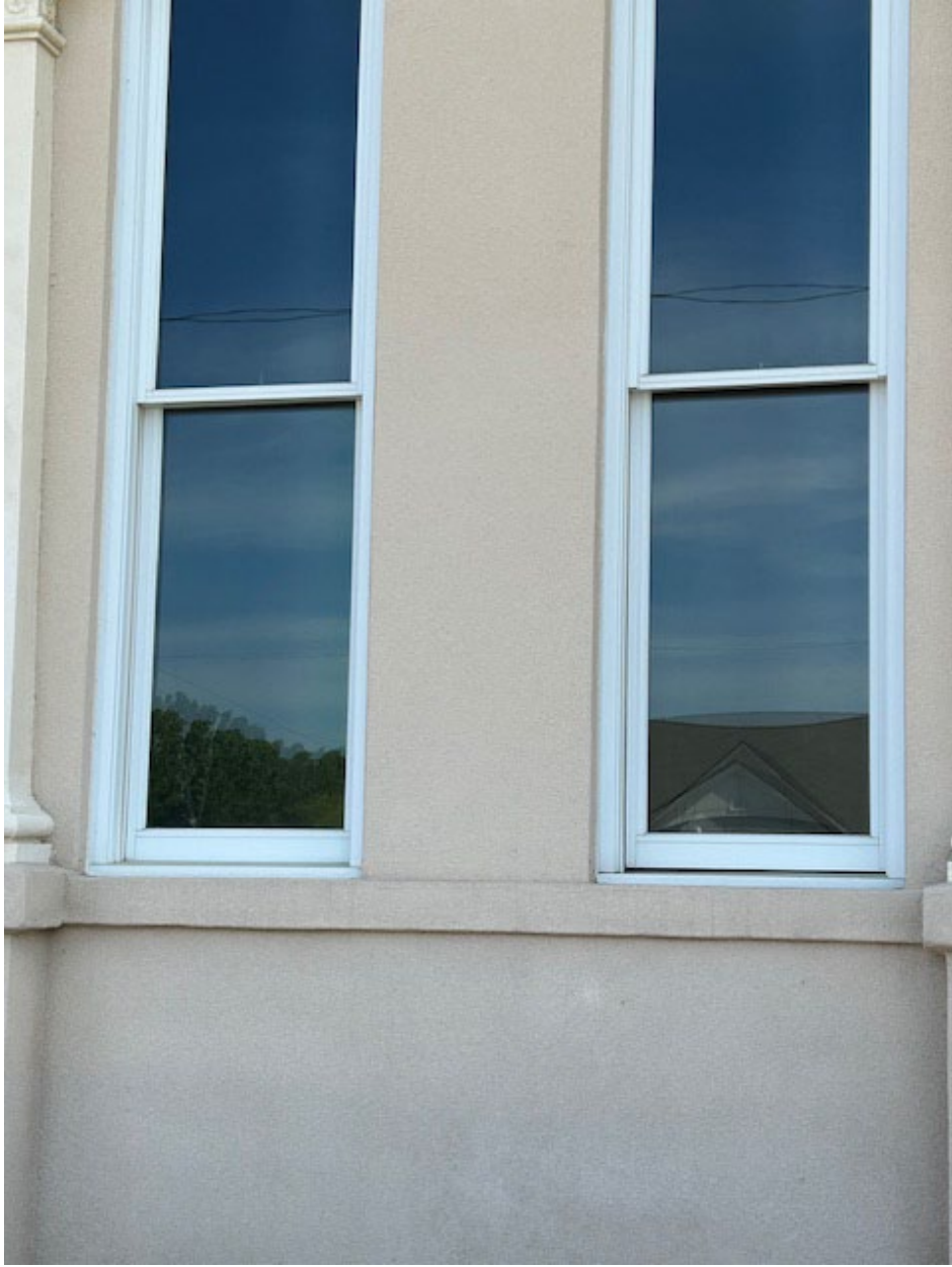
Gaps in bottom of windows
