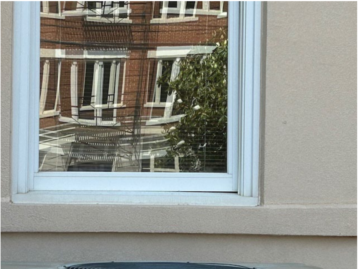
Gaps in bottom of windows
