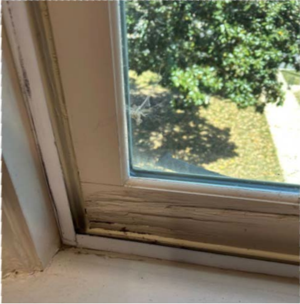
Interior wood damage due to deterioration
