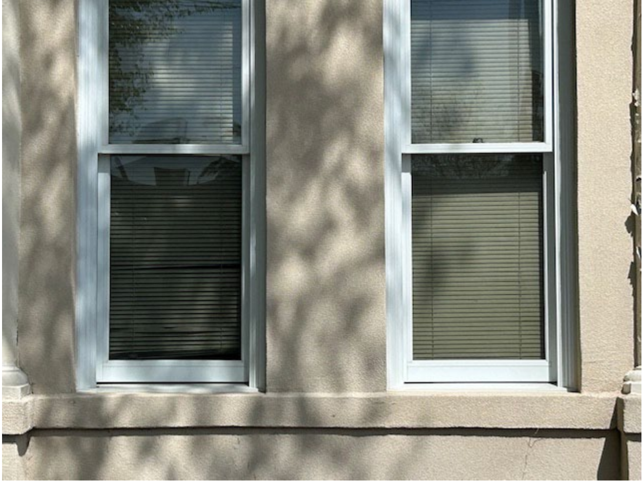
Gaps in bottom of windows
